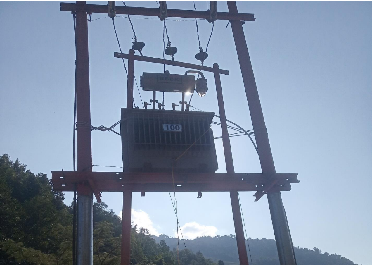
Figure 8: Transformer for construction power
